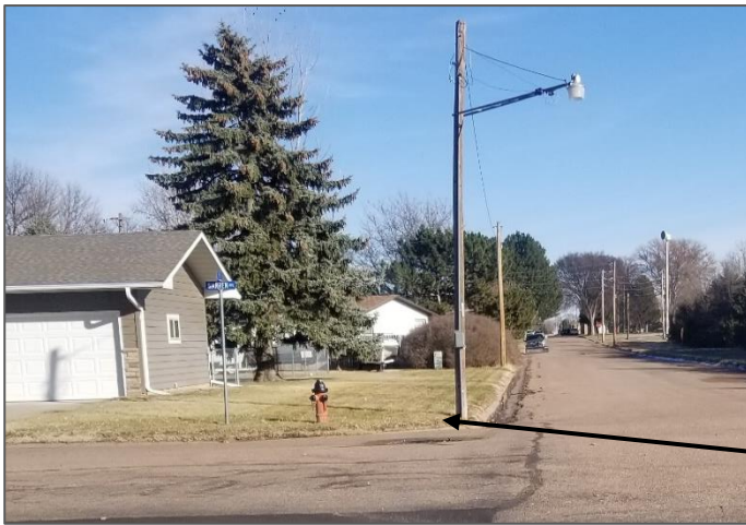
Intersection of 3 rd Street and Warren Avenue (facing east): lack of sidewalk and ADA accessible curb ramp.
